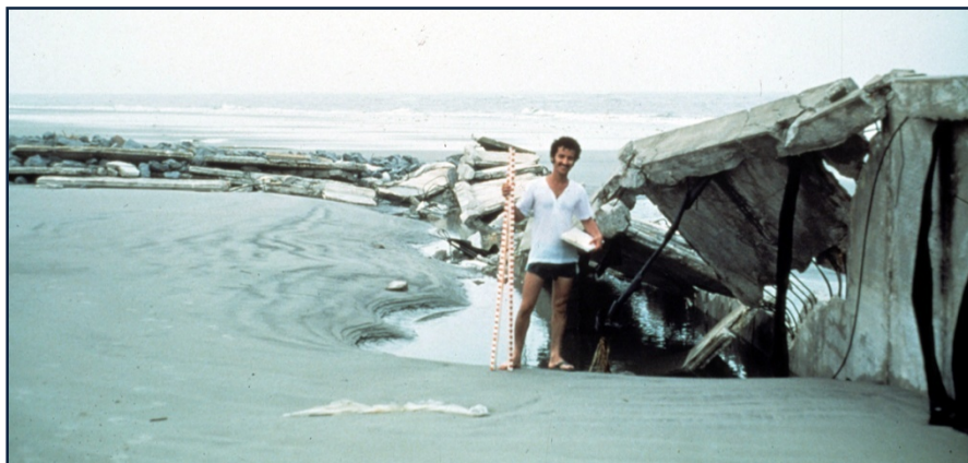
FIGURE T-6. Collapse of the concrete seawall at Renken Point in September 1979 during Hurricane David .
