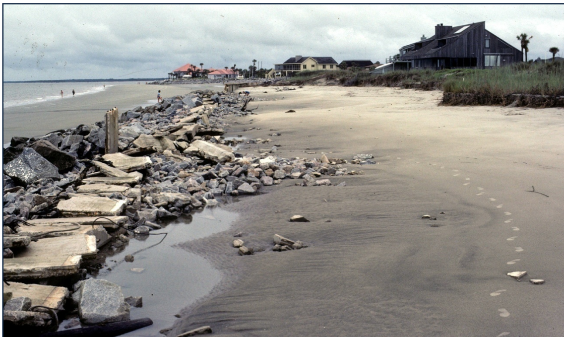
FIGURE T-8. [UPPER] Encroachment of the northern channel (deep blue area) of North Edisto Inlet and lack of maintenance leads to [LOWER] collapse of a section of seawall near Beach Court in 1983.
