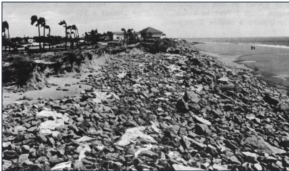
FIGURE 5.2.3a. Damages along Seabrook Island due to Hurricane David (5 September 1979). [UPPER] The concrete seawall and armor-stone “wingwall” at Renken Point on 7 September 1979. [LOWER] Collapsed riprap revetment south of the Beach Club on 5 September 1979. [Photos by WJ Sexton]
