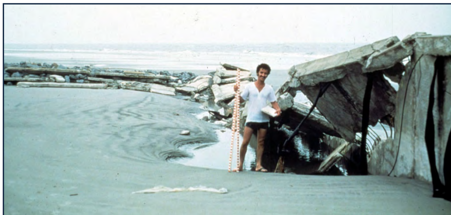
FIGURE T-6. Collapse of the concrete seawall at Renken Point in September 1979 during Hurricane David .
