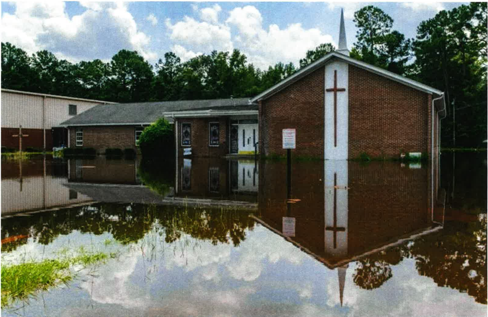
Floodwaters from the nearby Edisto River inundate Canaan United Methodist Church on Augusta Highway in Ridgeville on Aug. 10. At the time, the Edisto had reached nearly 17 feet, well above the major flooding stage at 15 feet.
